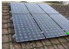
Connection to array frame.
