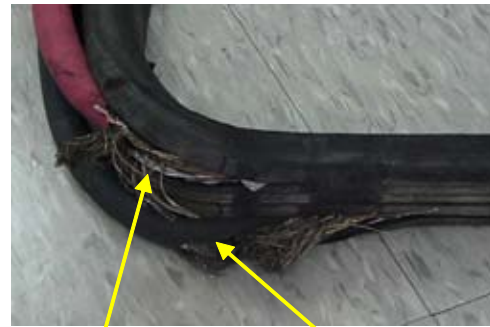
Broken cooling water pipe
